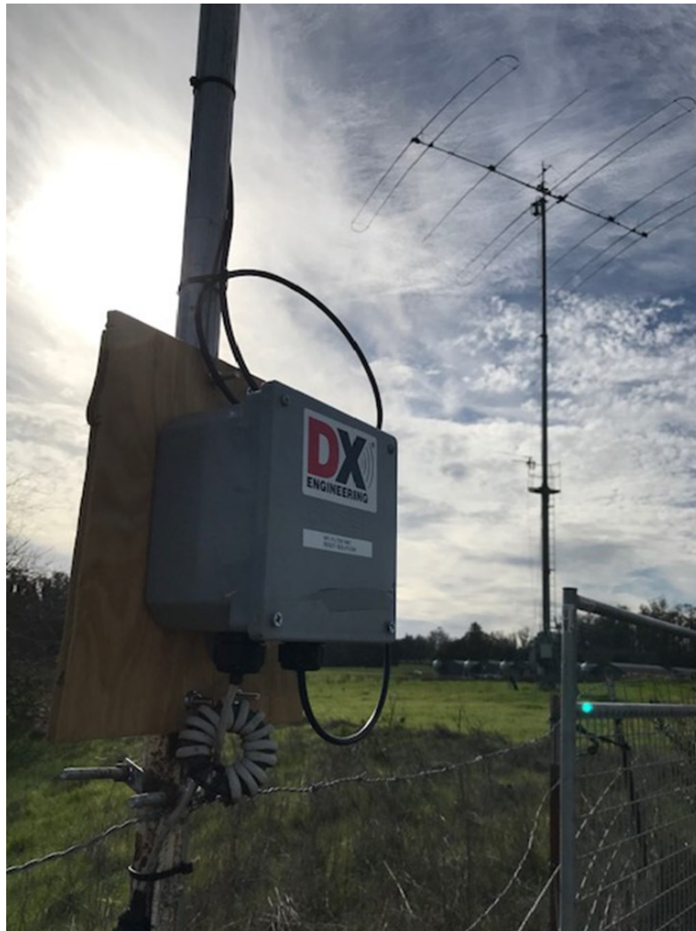
The completed filter installed. The 70' tower and DB42 are in the background
